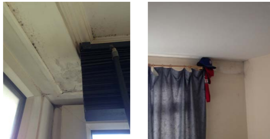
Mould and damp in the top corner of a room where there is a poor thermal barrier.
