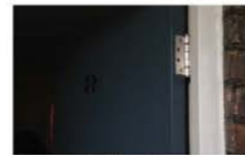
New doors don't fit well
