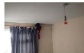
Mould growth at cold spots
