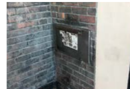
Rubbish chutes don't work for current needs.
