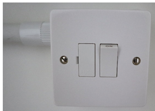
HRV Isolator Switch
