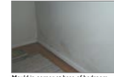
Mould in corner at base of bedroom wall of flat with communal stairwell
