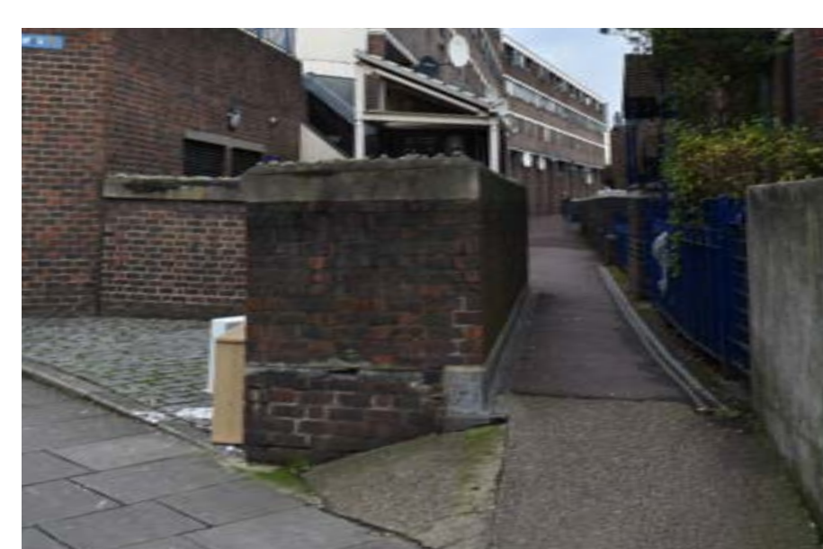
Designated area for large rubbish collection has steep narrow access.
