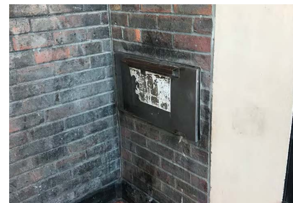
Rubbish chutes don't work for current needs.
