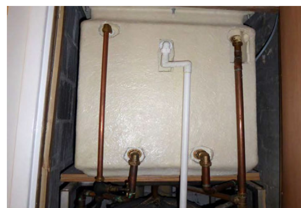
Existing water tanks are rusted.
