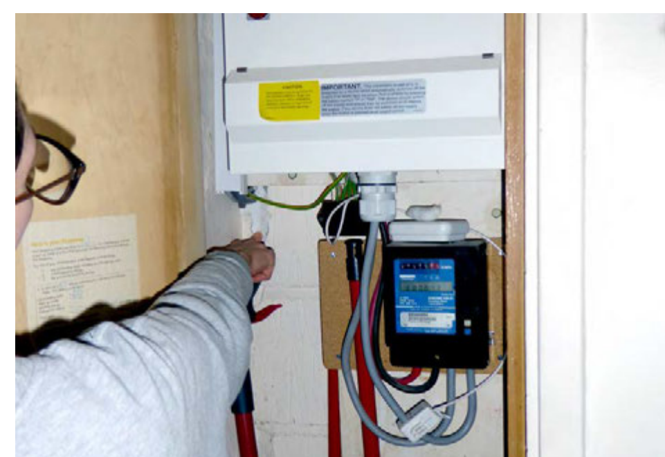
Electrical installation needs replacement
