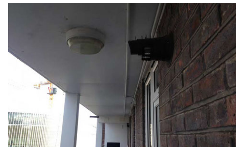
Homes have individual boilers
