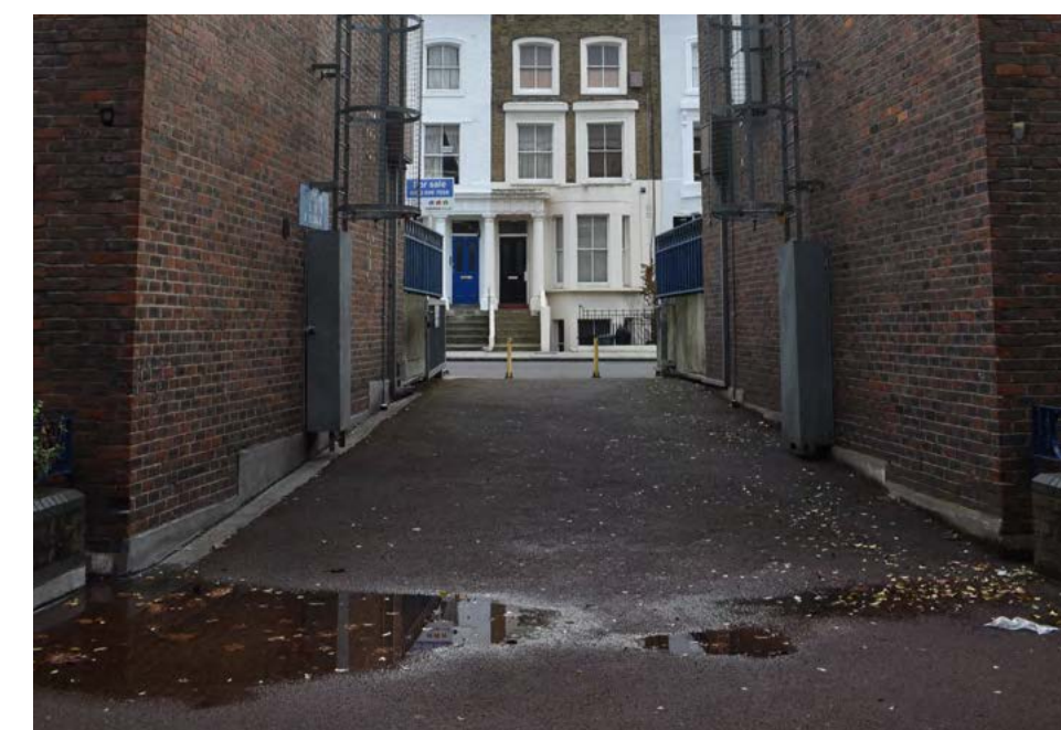
Walkway constantly floods
