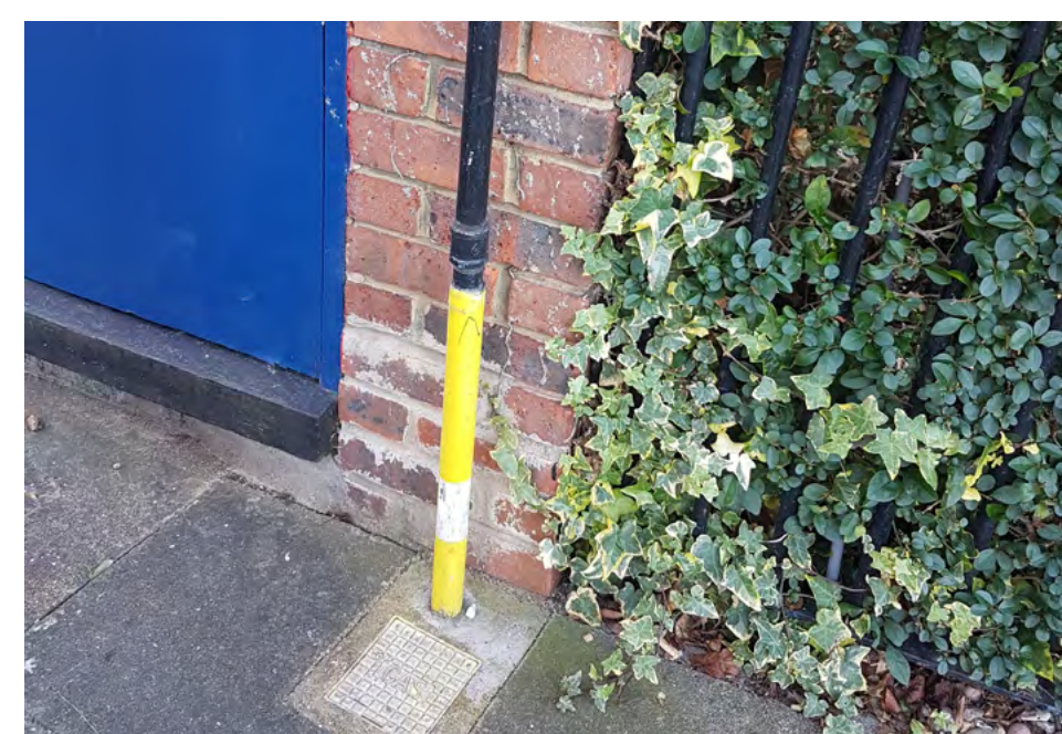
Exposed gas pipes
