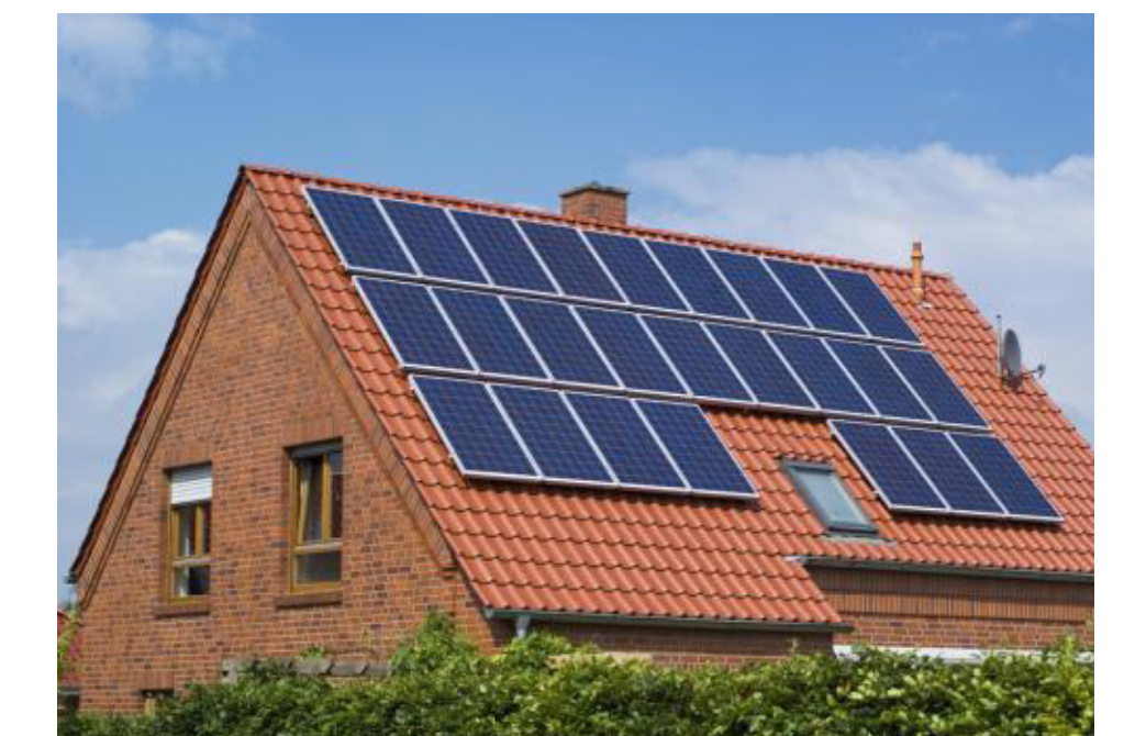
PV solar panels on roof: reduce energy bills
