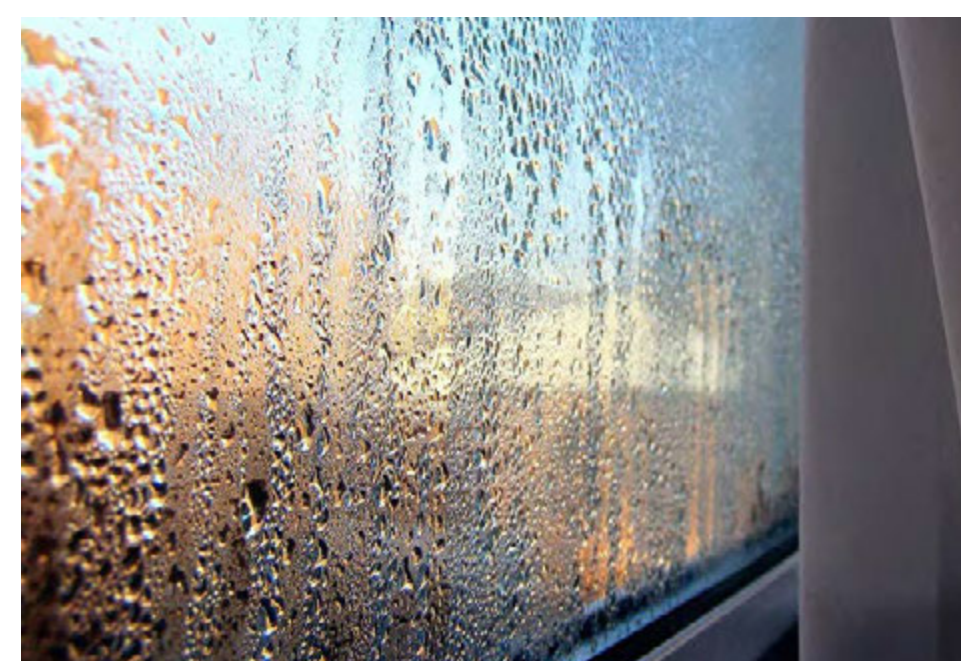
Condensation on windows and walls
