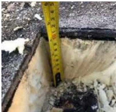
Lack of insulation in existing walls and roofs
