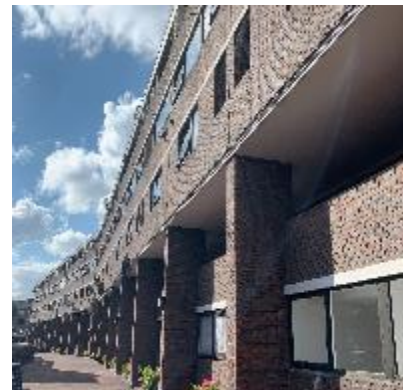
Thermal Bridging issues – causing damp and heat to escape
