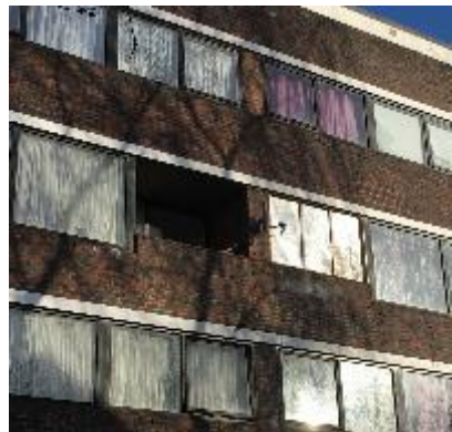
Single-glazed windows – causing condensation and draughts
