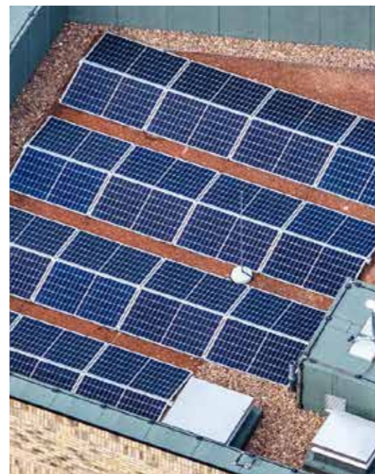
▲ Indicative arrangement on a flat roof. Panels are angled to achieve maximised sunlight absorption for the specific building.
