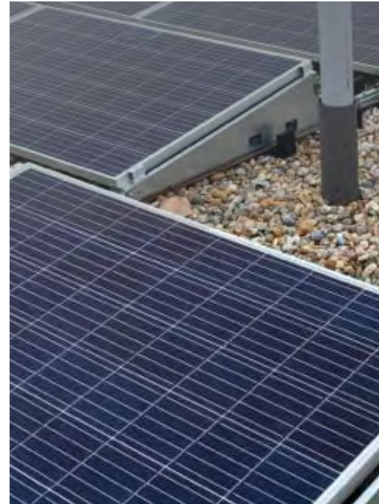
▲ Typical PV panel
