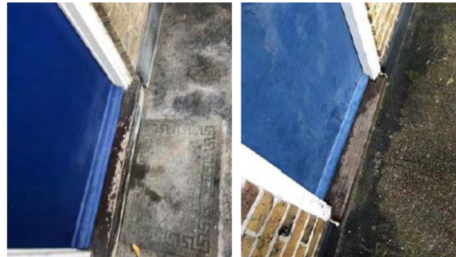
Figure 105 - Condition of area around existing door cills
