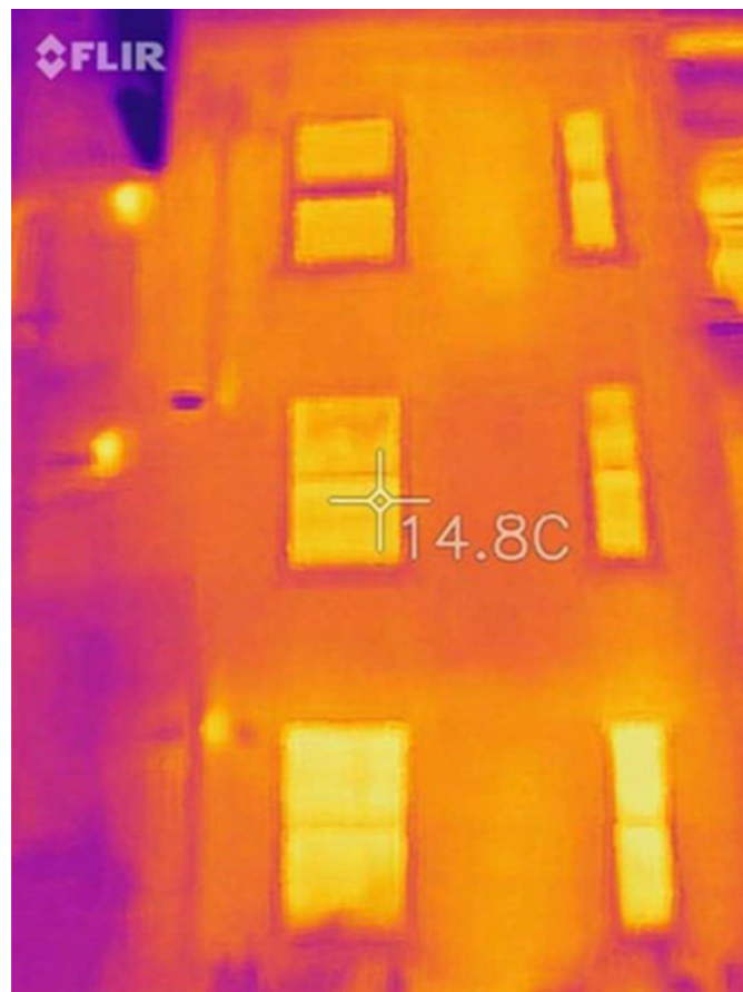
Figure 56 - Thermal Imagery of Morland House showing heat loss through facade (red/orange area)
