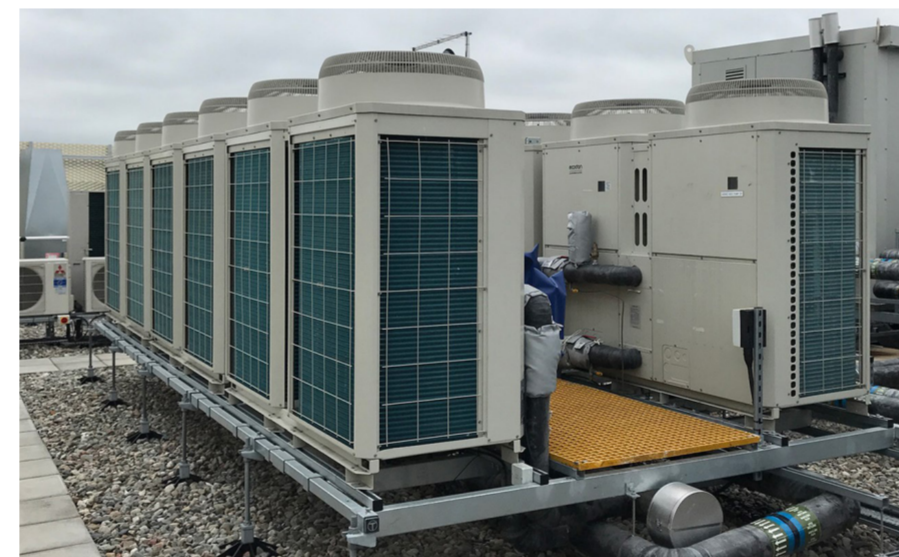
Air source heat pump condenser units
