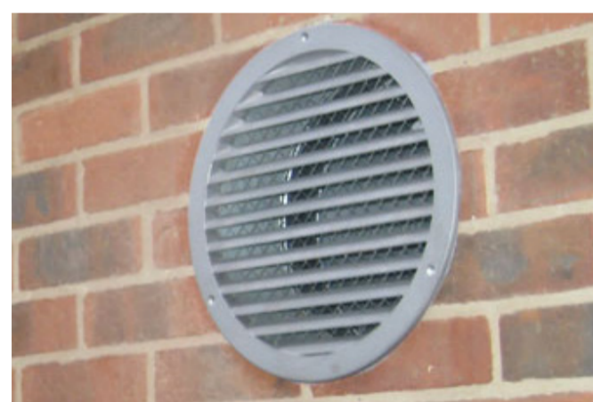
MVHR air intake/ extract grille on outside of building
