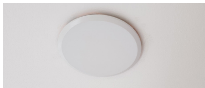
Above: ceiling mounted sprinkler
