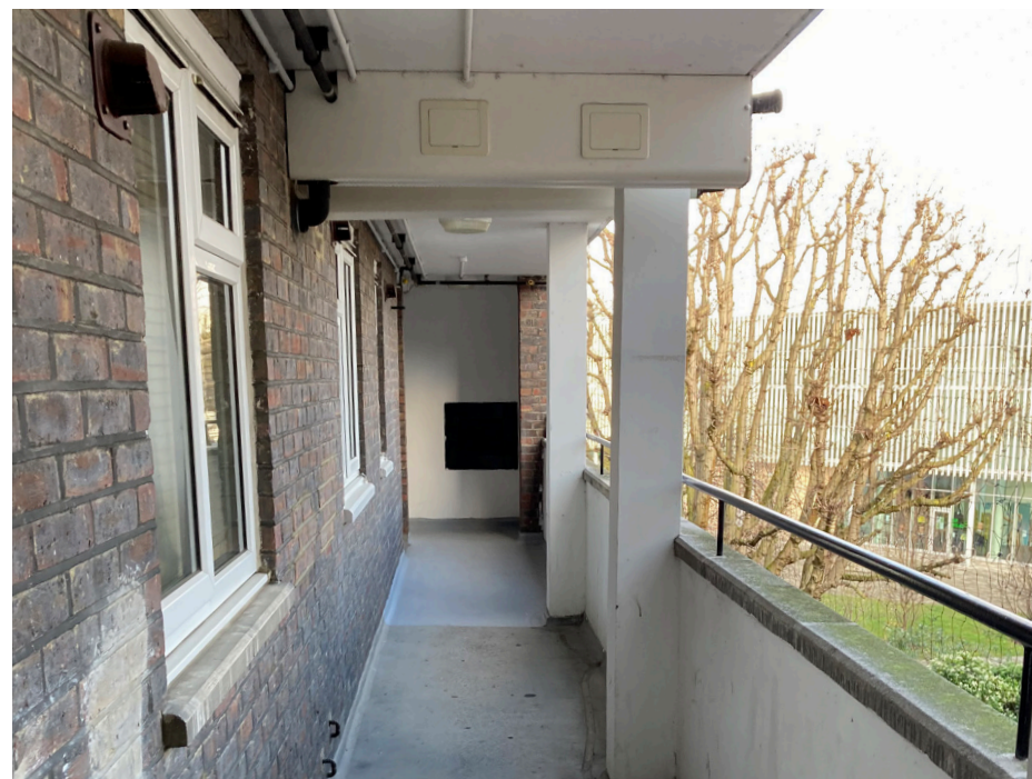
Figure 24 - Boiler flues to soffit of deck access
