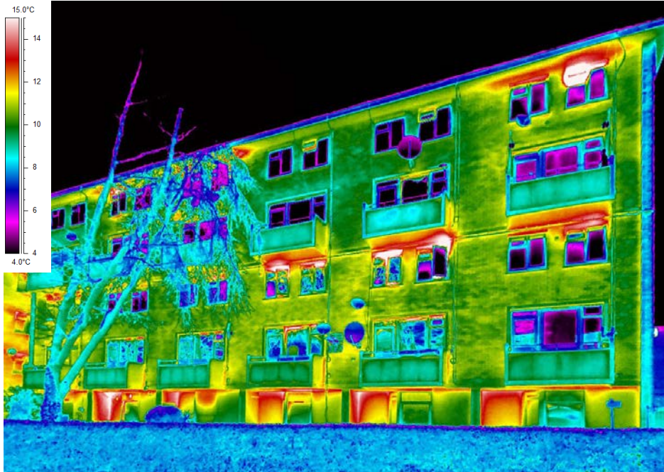
Figure 20 - Thermographic image of south facade of east wing, showing significant heat loss through balcony slabs and at edge of roof - Survey date 16/03/2021
