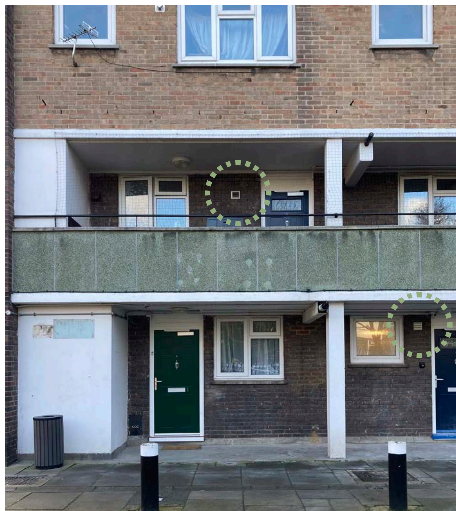
Figure 61 - Extract fan grilles on external wall
