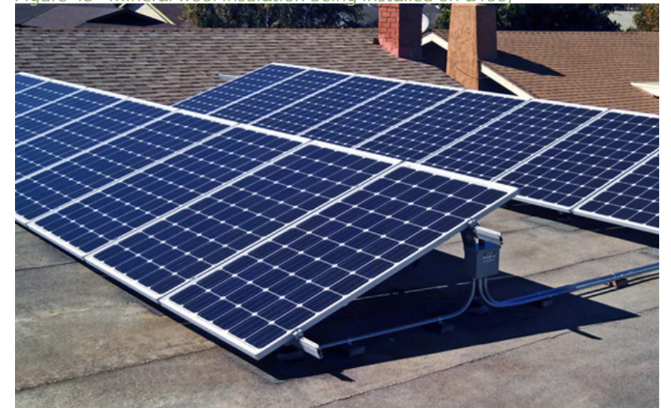
Figure 49 - Photovoltaic panels on flat roof
