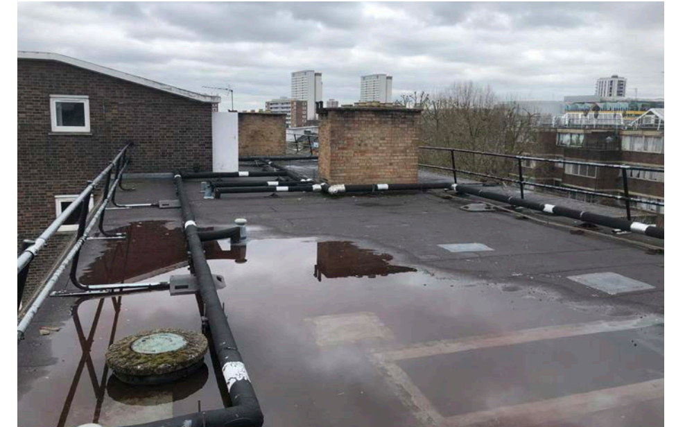
Figure 27 - Gas pipes running across rooftop
