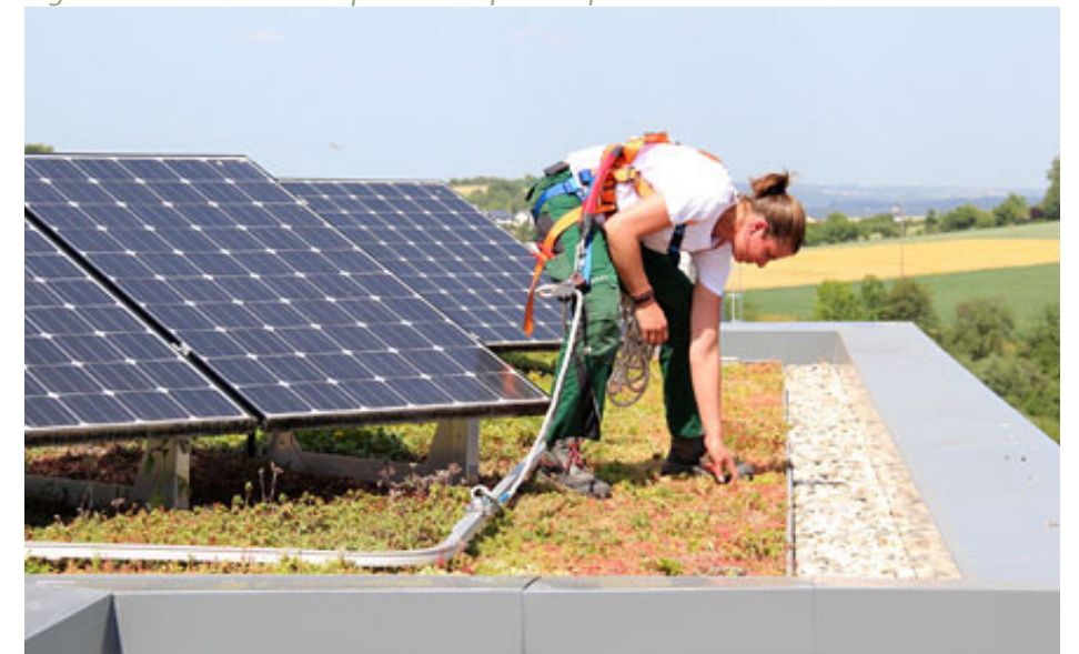
Figure 50 - Photovoltaic panels on green roof
