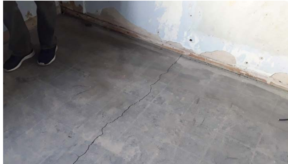
Figure 10 - cracking to floor screed, overhang maisonette floor
