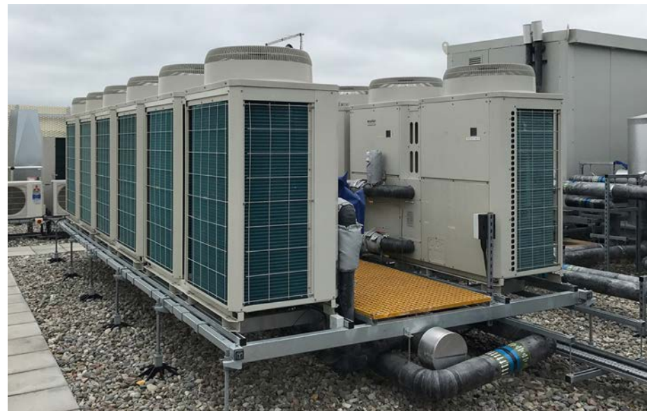
Figure 51 - Communal air source heat pump
