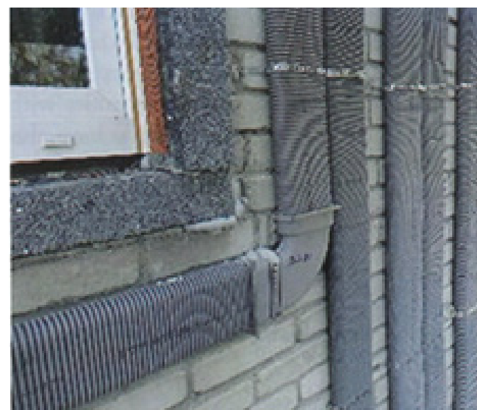
Figure 63 - External ductwork runs prior to application of external wall insulation. This would be used with a communal system
