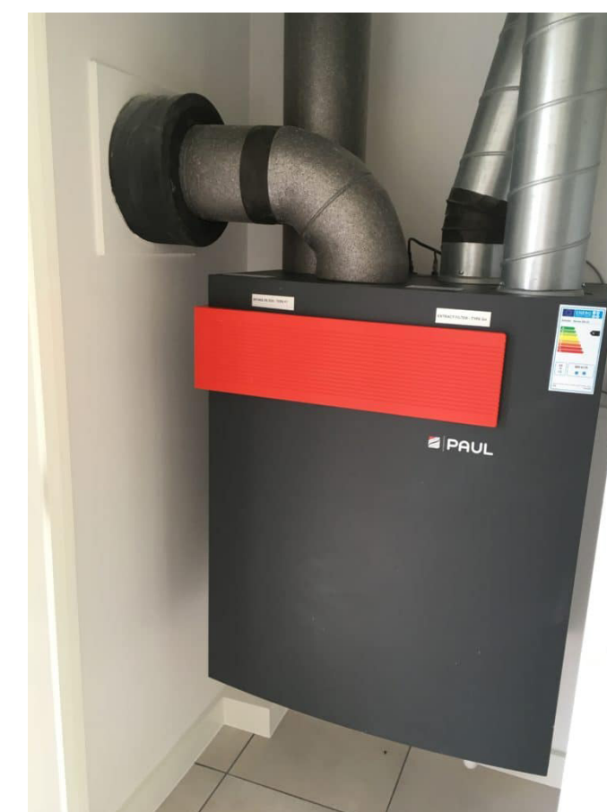
Figure 60 - MVHR unit with insulated exhaust & intake ducts and uninsulated, metal extract & supply ducts
