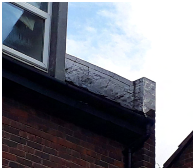
Figure 19 - Poorly maintained parapet to gable end wall
