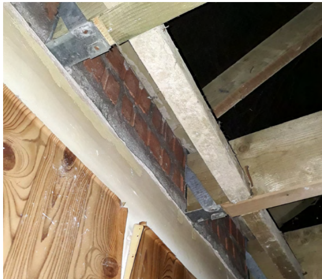
Figure 18 - First floor joists on metal hangers (here at eaves of lean-to roof)
