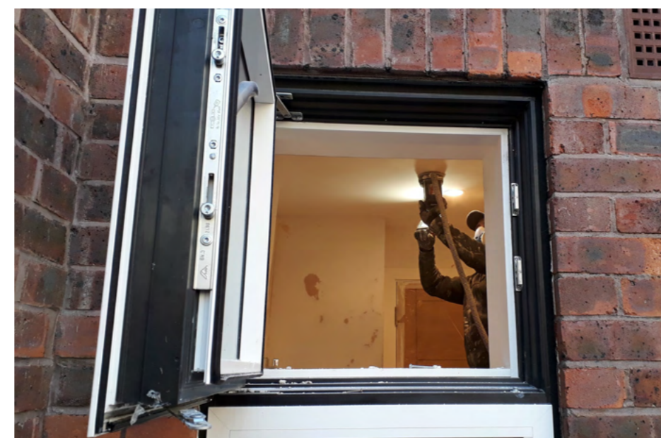
Figure 65 - New side hung triple glazed casement window at 50 Verity Close. The frame is deep, but appears slender from inside & out
