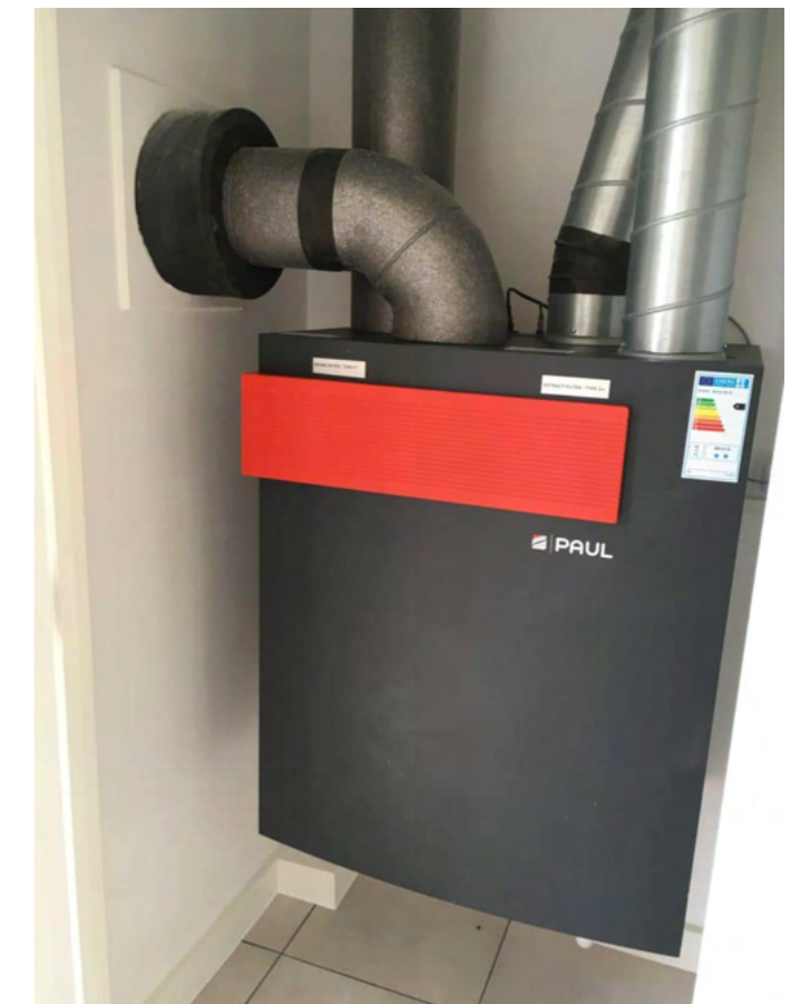
Figure 63 - MVHR unit with insulated exhaust & intake ducts and uninsulated, metal extract & supply ducts
