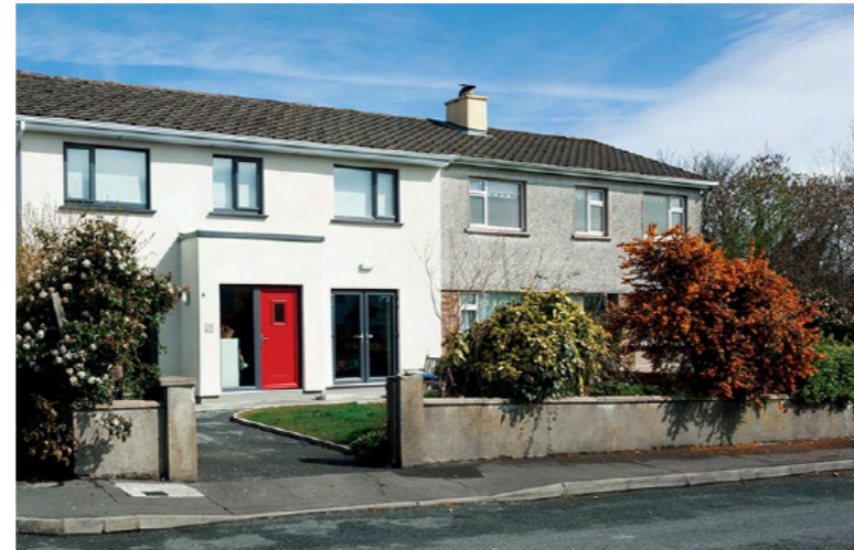
Figure 45 - Rendered EWI completed retrofit scheme Note: other finishes, including brick slips to replicate existing are possible
