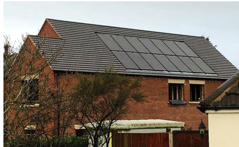
Figure 74 - Photovoltaic panels installed in line with roof covering
