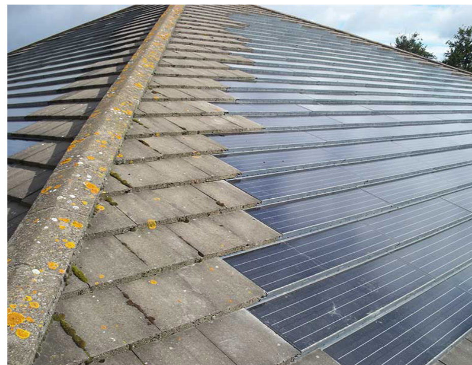
Figure 75 - Photovoltaic tiles among existing tiles
