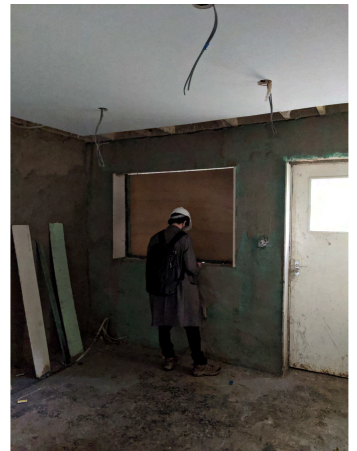
Figure 32 - 50 Verity Close - Diathonite plaster applied to inside of walls (greenish hue is reinforcement mesh)
