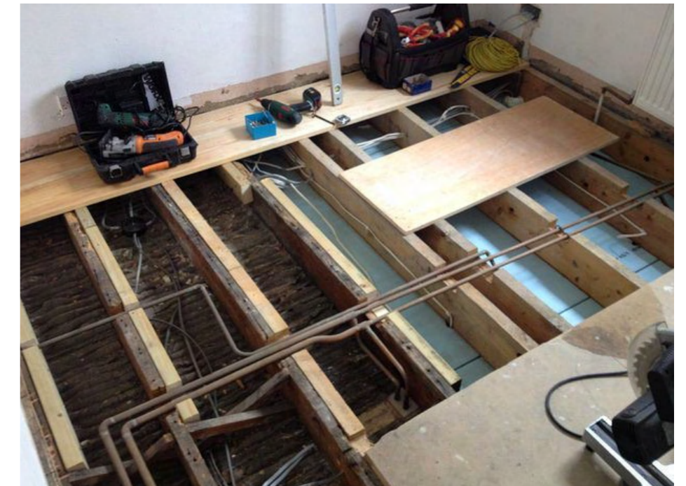
Figure 80 - Floorboard temporarily removed to allow insulation to be fitted between joists and for better fixing of floorboards to reduce squeakiness
