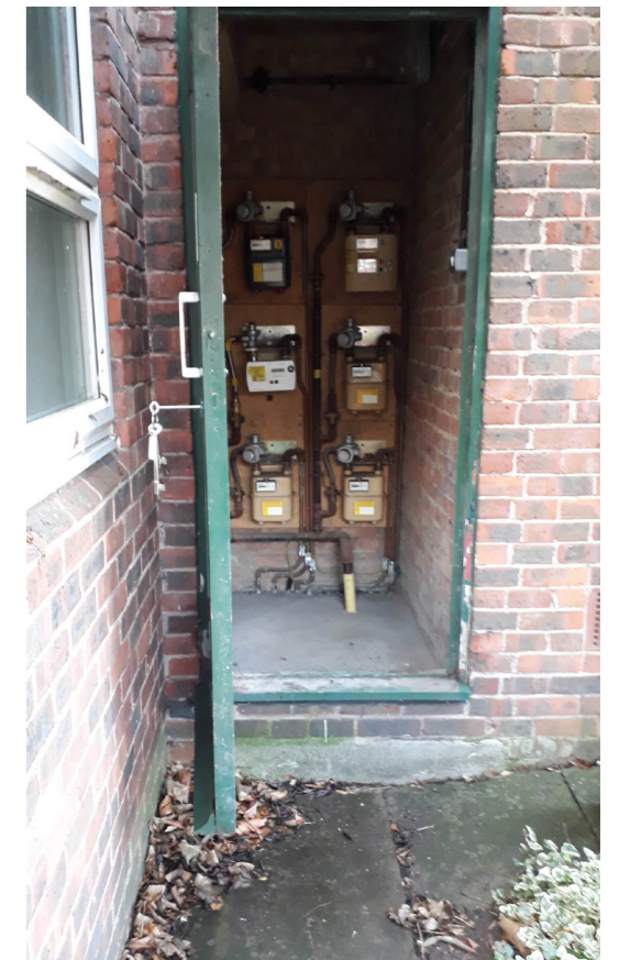
Figure 85 - Inside existing gas meter room
