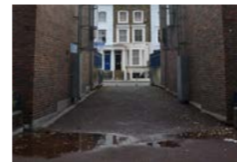
Walkway constantly floods
