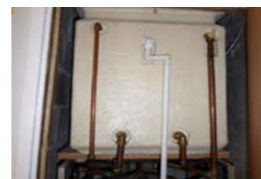
Existing water tanks are rusted.
