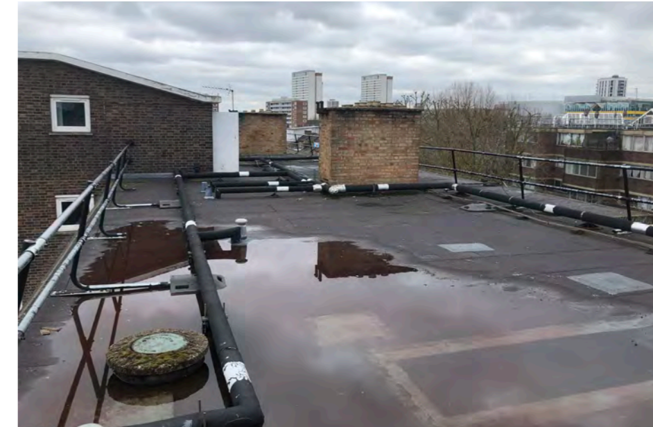
Figure 34 - Gas pipes running across rooftop
