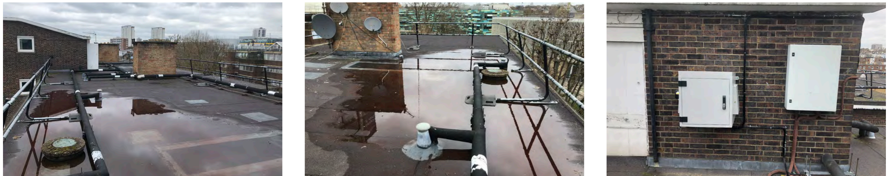
Figure 20 - West wing roof conditions
