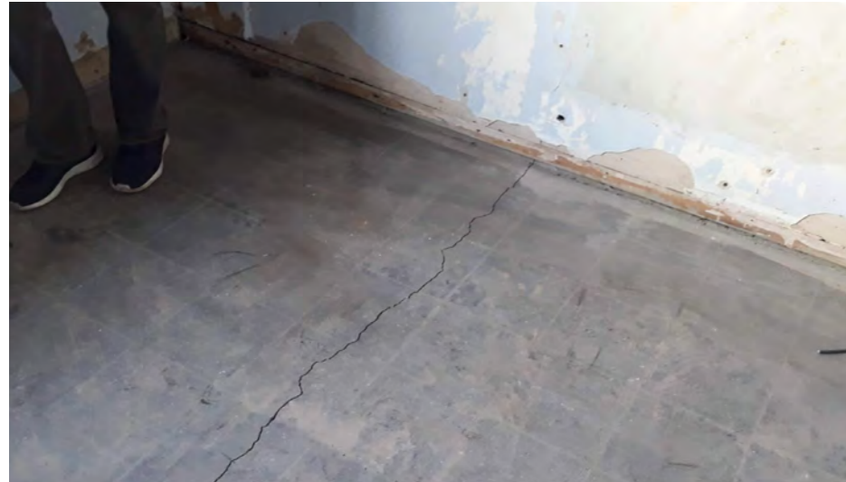
Figure 11 - cracking to floor screed, overhang maisonette floor
