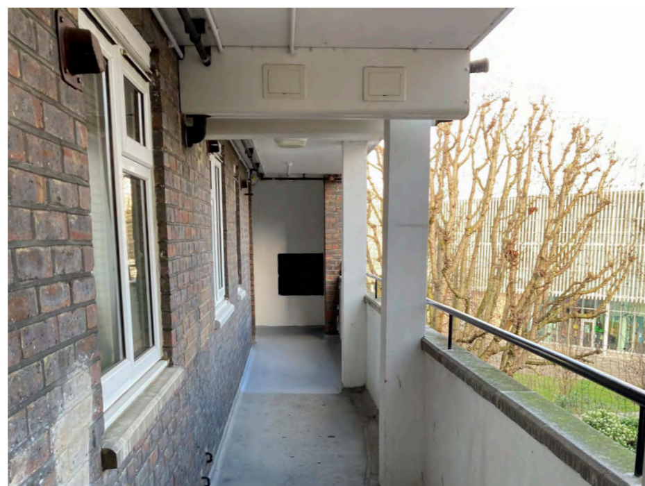
Figure 31 - Boiler flues to soffit of deck access
