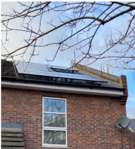
Figure 24 - Photovoltaic panels to the east side of the roof
