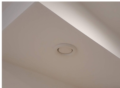
Figure 19 - Air supply fitting in ceiling
