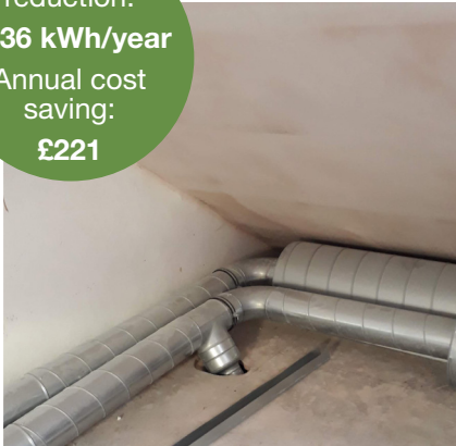
Figure 20 - Fire-rated ductwork, prior to boxing-in
