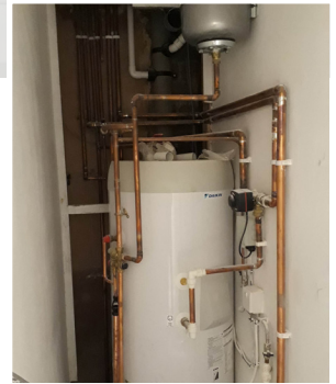
Figure 23 - Hot water tank & pipework in under-stairs cupboard
