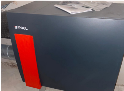
Figure 21 - MVHR unit in roof space
