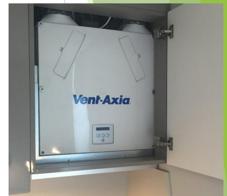
Unit inside cupboard
