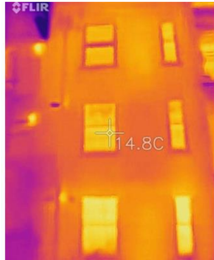
Walls have poor insulation, allowing heat to escape from the home
