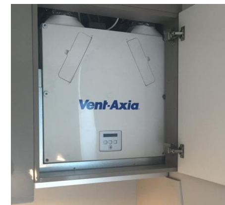
MVHR unit inside cupboard
