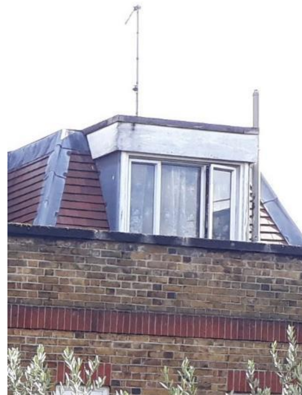
Roof has poor insulation, which allows heat to escape
