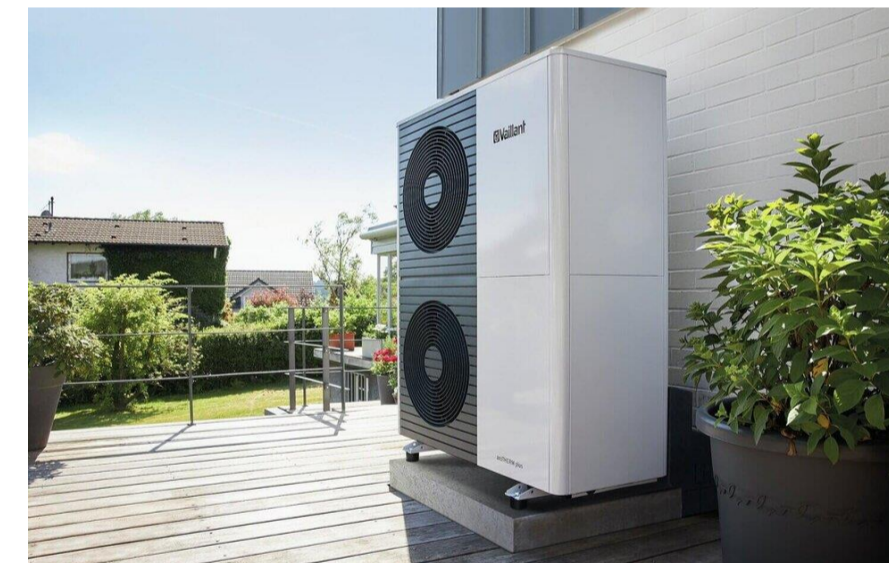
Air source heat pump condenser units
