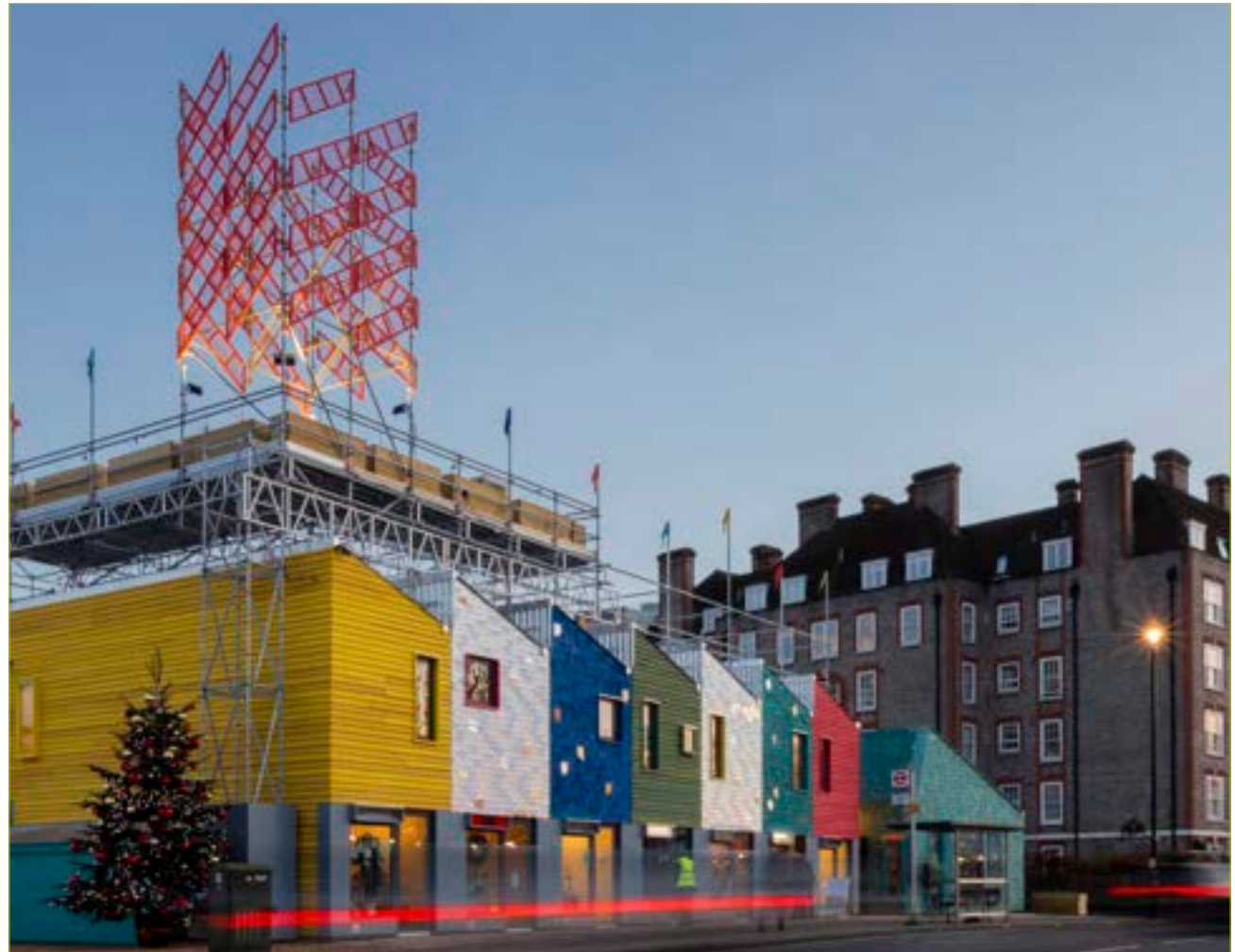
Ebury Bridge Estate by Jan Kattein Architects, ARUP; Gardiner + Theobald; Meanwhile Space CIC - Case Study from the Playbook of Ideas Image © JKA
