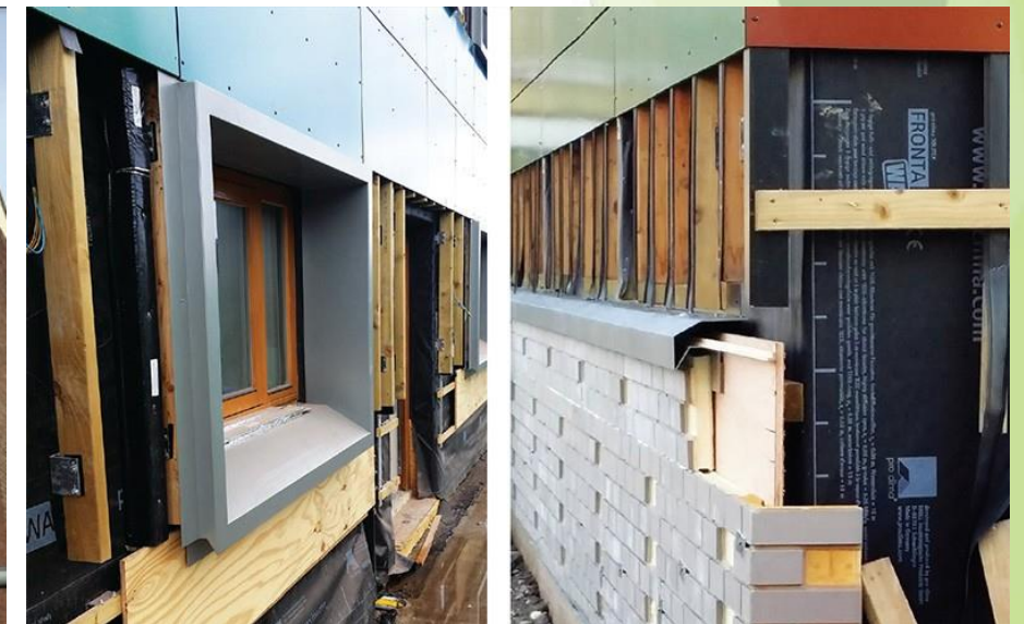
New triple glazed balconies, new external wall insulation, Rockpanel and Gebrick cladding.
