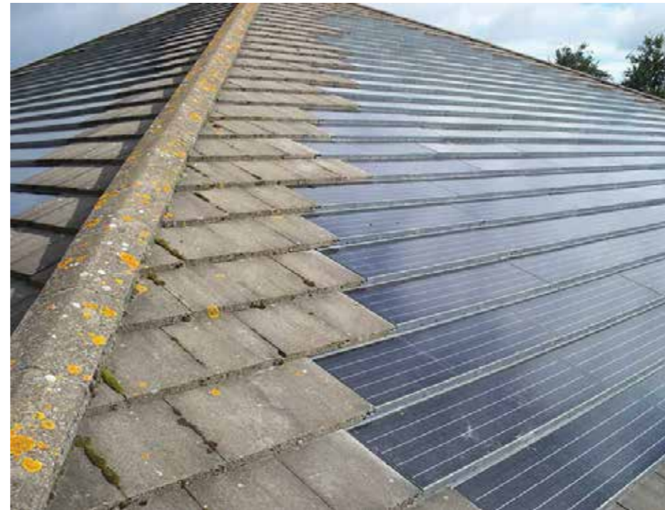
Figure 43 - Photovoltaic tiles among existing tiles
