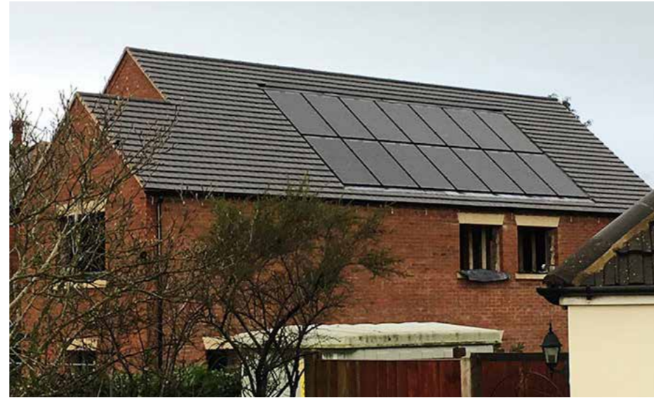
Figure 42 - Photovoltaic panels installed in line with roof covering
