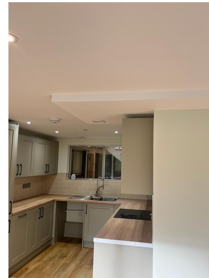
MVHR metal ductwork
