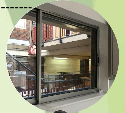
Fire rated entrance doors & windows into atrium
