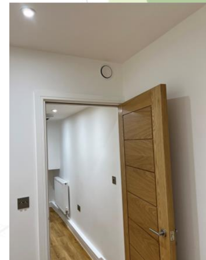
MVHR plastic ductwork
