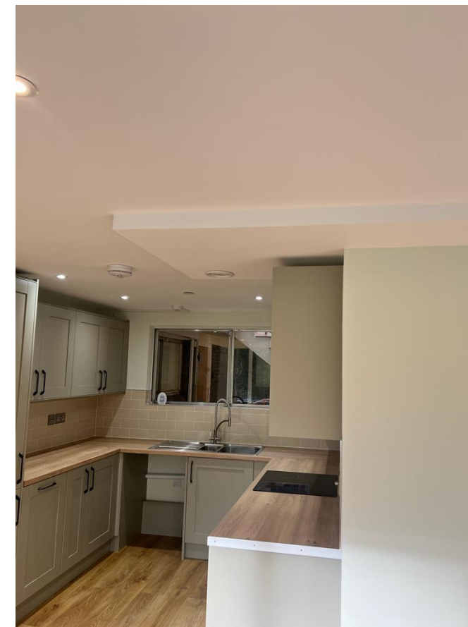
MVHR metal ductwork
