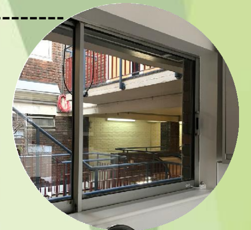
Fire rated entrance doors & windows into atrium
