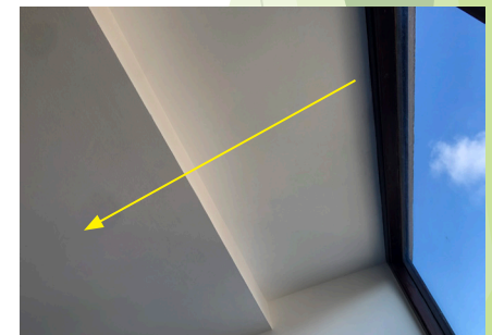
02: New dropped ceiling and the set-back from the window. This will be much deeper into the room with an inward swing.
