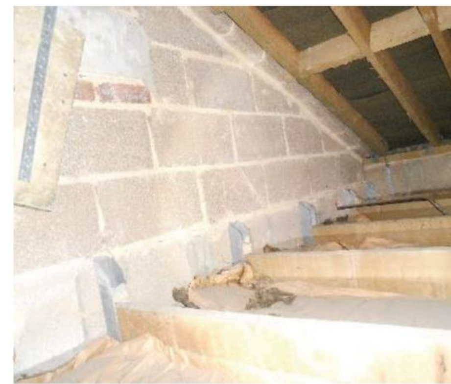
Poorly Insulated roof
