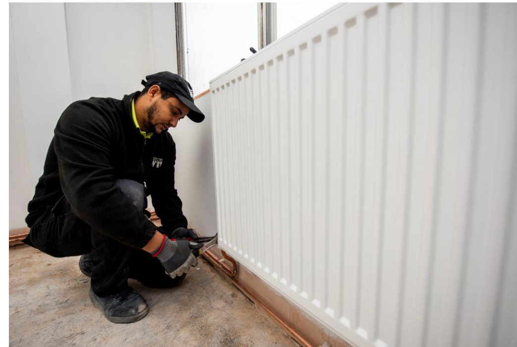
New Radiators + Pipes Existing radiators will be replaced with a similar type.
