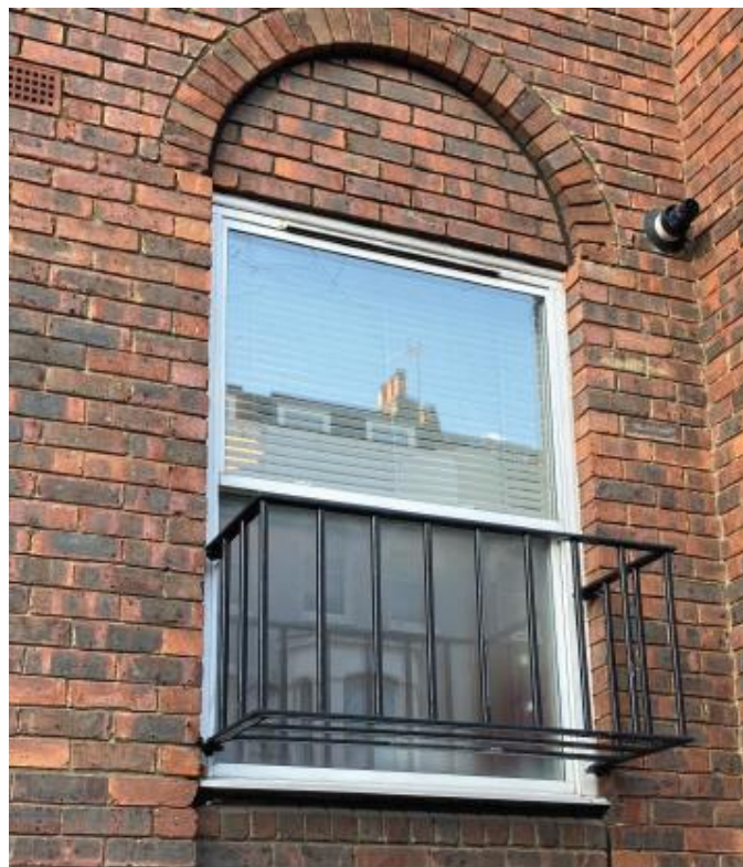
Double glazed sash windows that do not perform well
