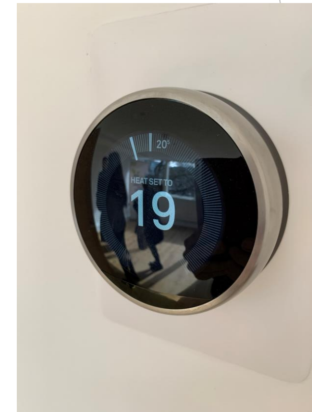
Thermostat Controls for heating.
