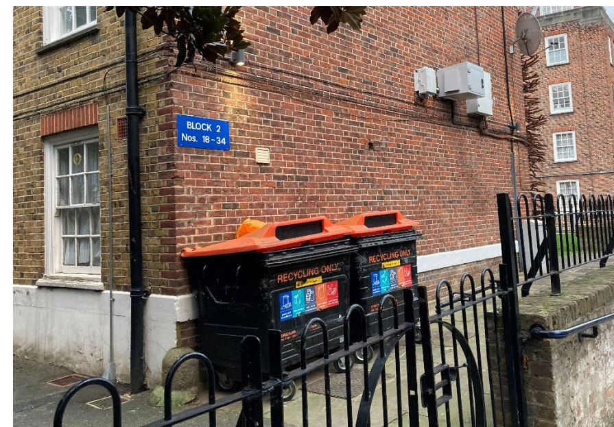
Existing recycling bins at flank wall, additional required to remove bin chutes
