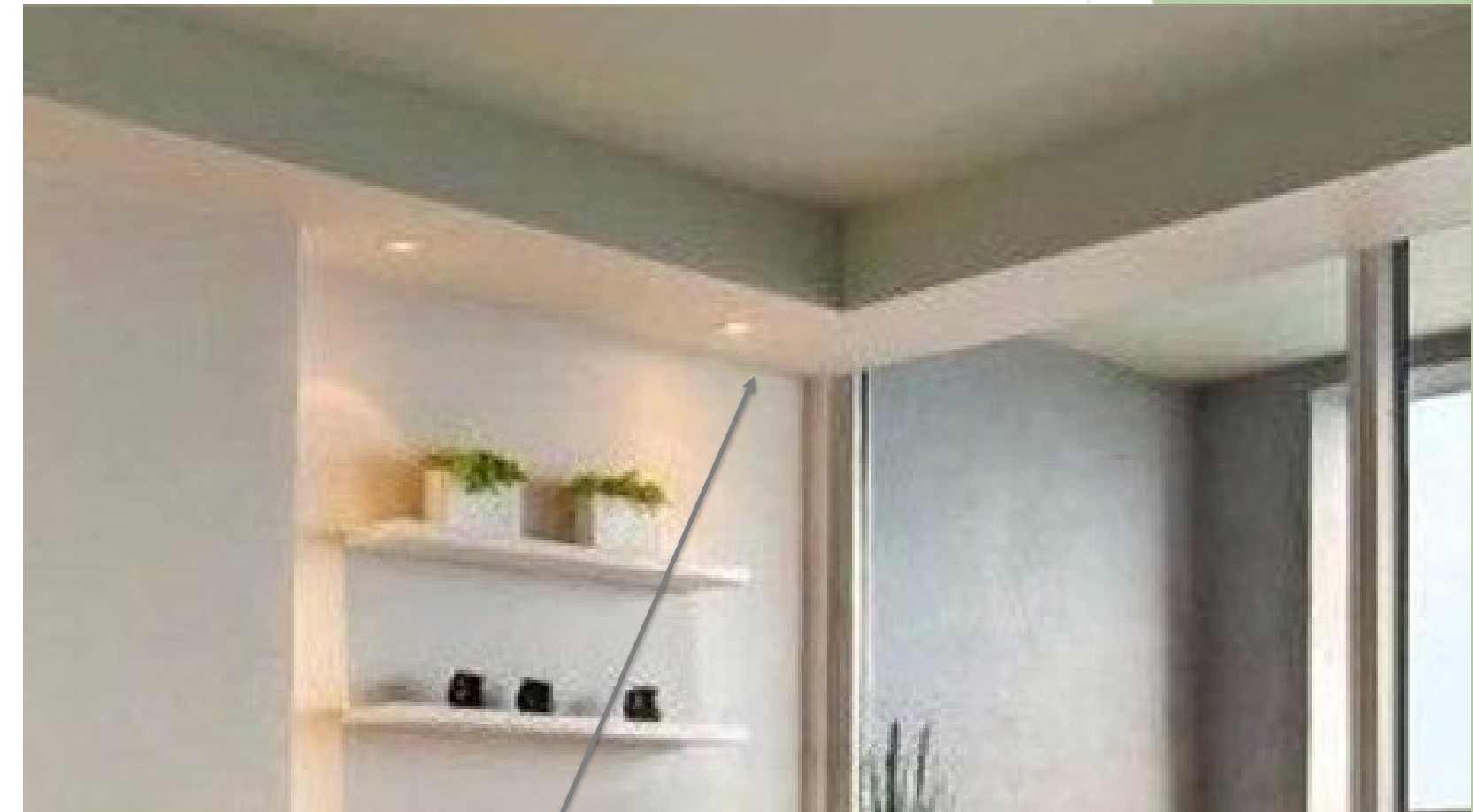
This is an example of a bulkhead where a section of the ceiling that has been dropped to conceal MVHR ducting which has been boxed-in or enclosed
