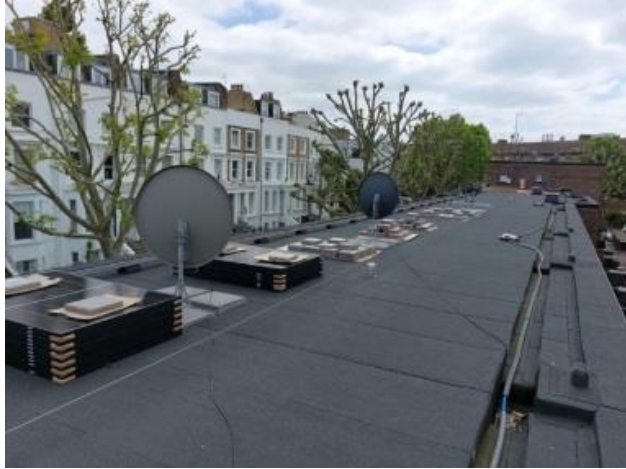
Camelford Court solar PV
