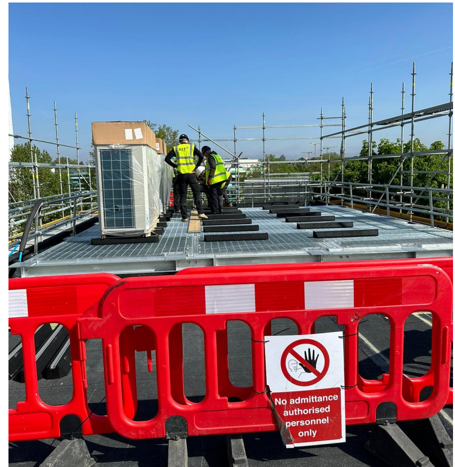
Image 4: picture of air source heat pumps being installed at Treadgold House in May 2024.
