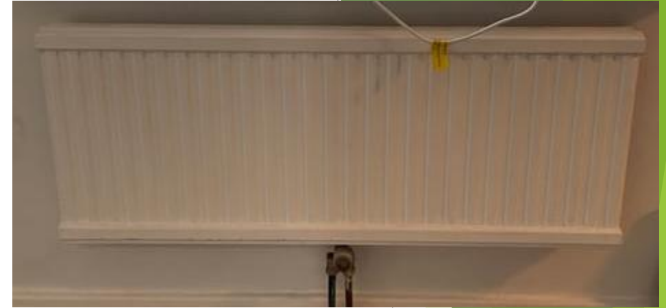
Originally Installed Radiators in 1960s
