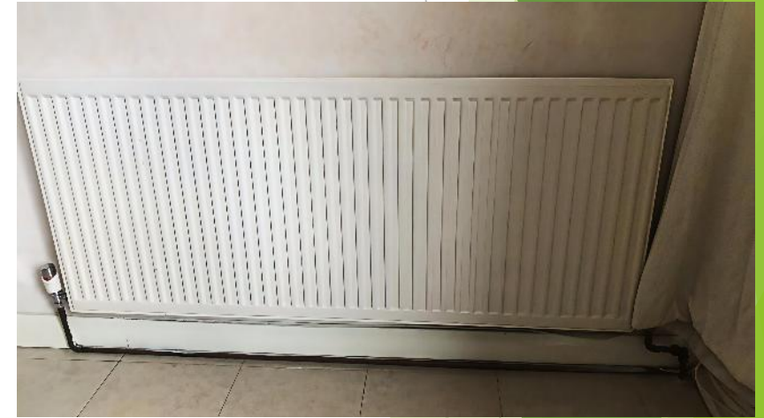
Various replaced and added radiator through years
